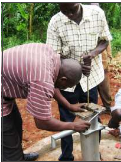
Men installing the finishing touches on a well at Rapha School in Jinja, Uganda
